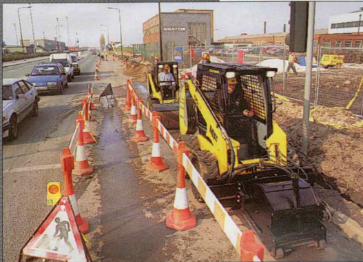
The MF516XP and planer make a highly effective but compact tool for pavement and carriageway repairs.
